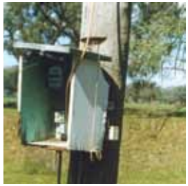
Defective Meter Box
