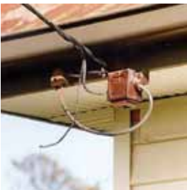
Defective Service Fittings
