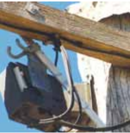
Defective Point of Attachment
