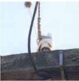
Defective, Cracked or Chipped Insulators
