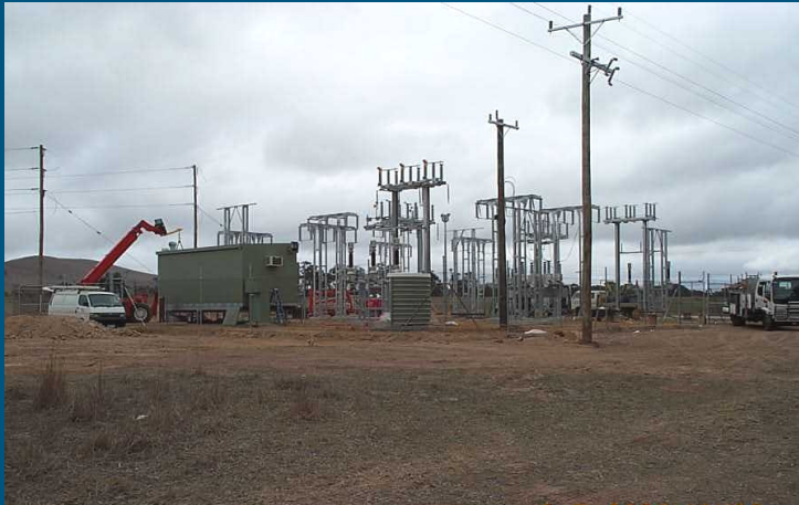
The new control room
